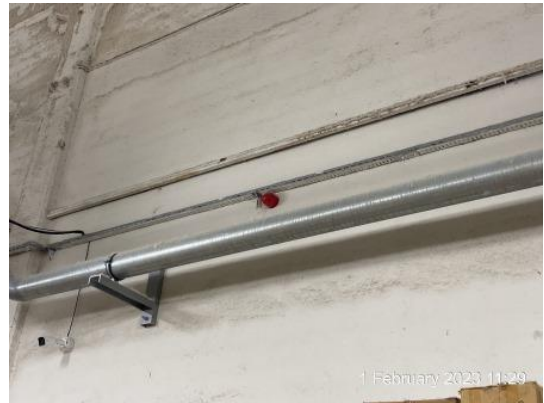
Visual alarm at weaving area.JPG
